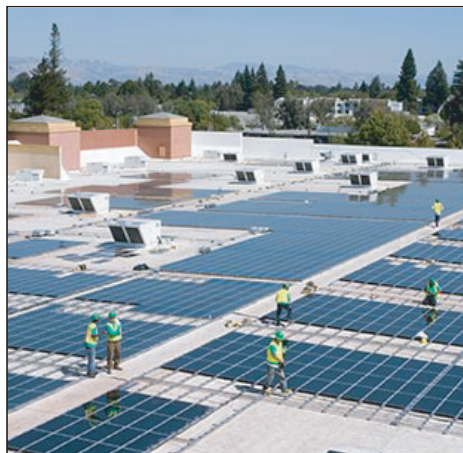
Solar panels on Walmart rooftop.
