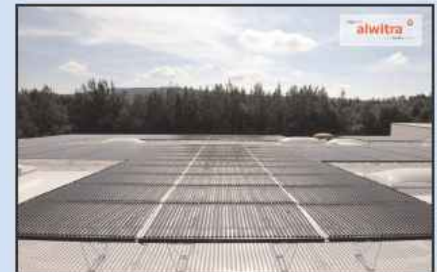
p50 Solyndra's CIGS photovoltaic arrays on alwitra's roofing.
