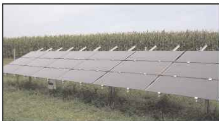
An installation of MiaSolé's modules.
