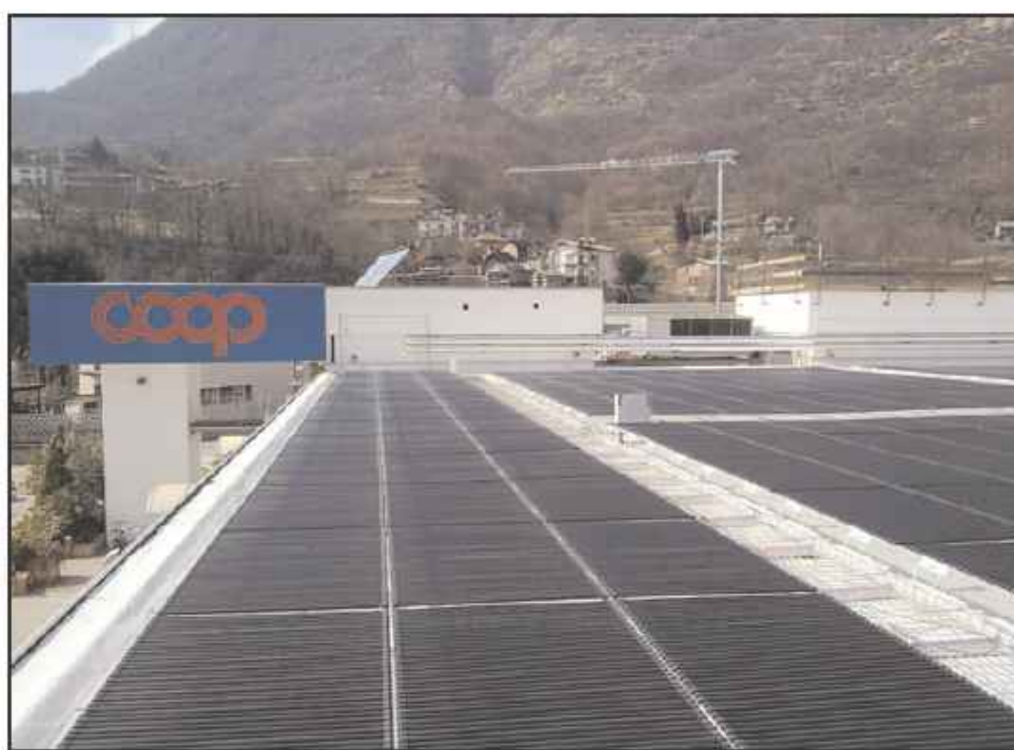
Solyndra CIGS PV installation at Nova Coop, Villa Dossola
