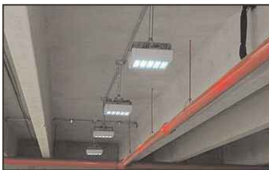
LED lighting in parking garage at the Universities at Shady Grove.
