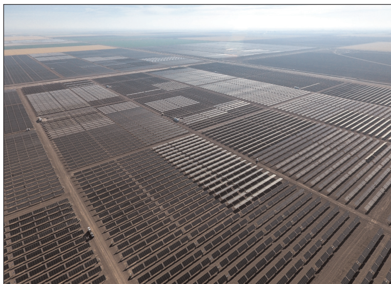
Solar Frontier Americas' Midway I & II solar plants in the Imperial Valley of Southern California.
