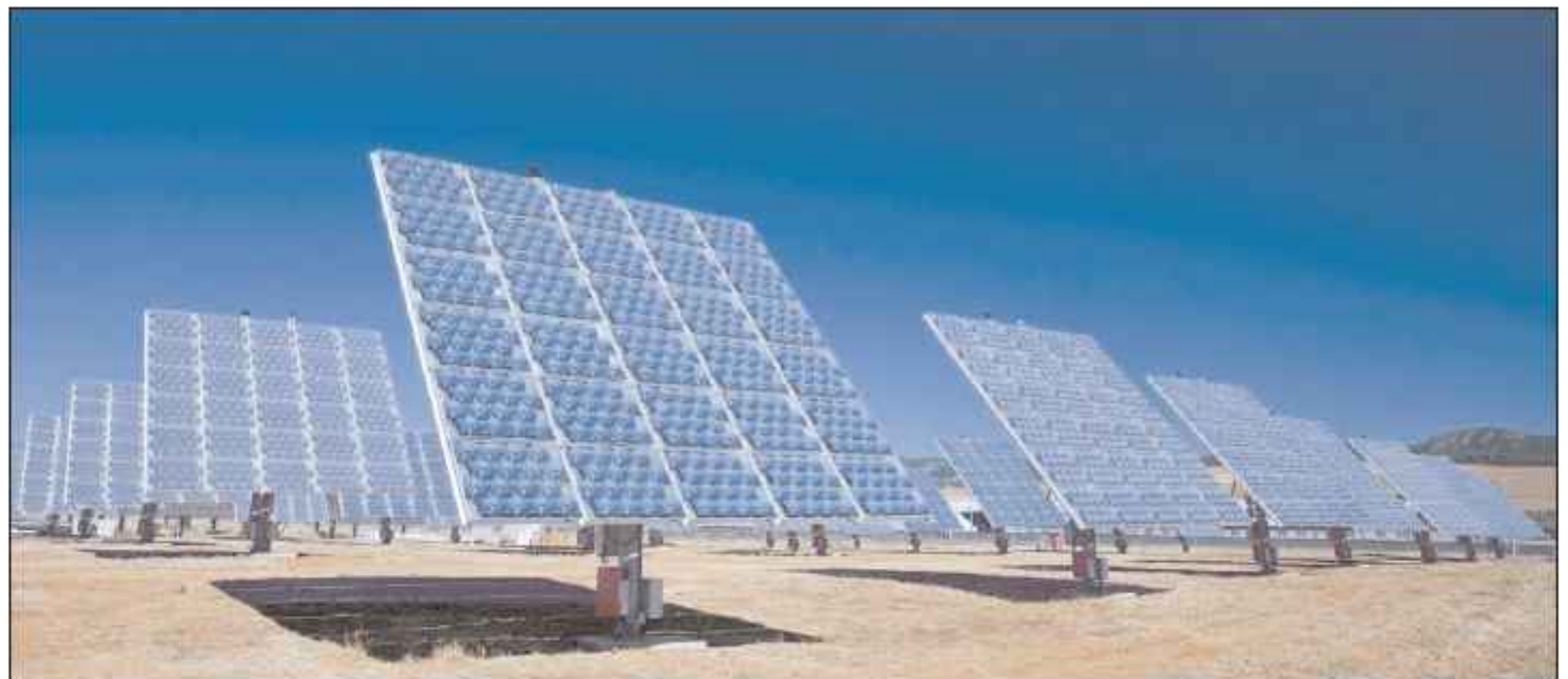
Solfocus existing CPV systems at the ISFOC installation in Puertollano, Spain.
